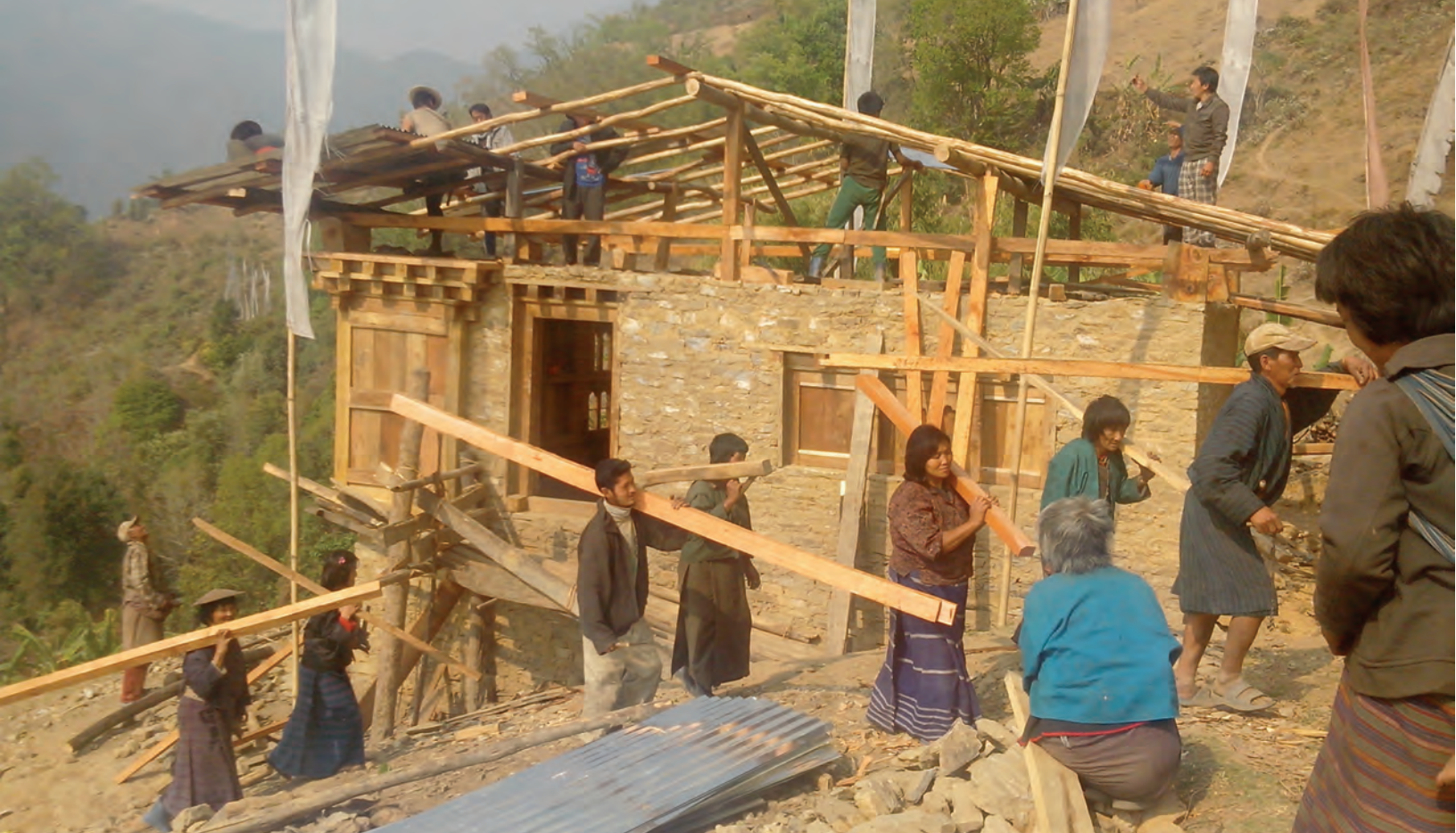
Community members of Dak, Monggar working at the construction of Ap Leki's house
